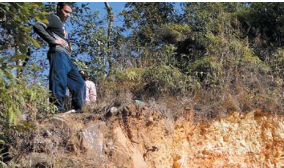
Photo 40: Landslide triggered by on-going road construction
