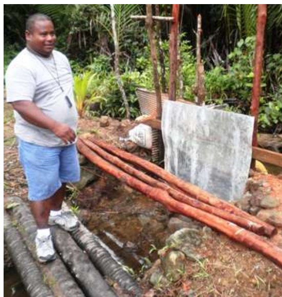
Figure 8: A simple flood gate installed at Ngmis
